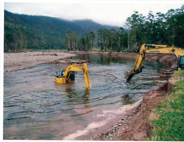
Cleaning up after 2007 floods
