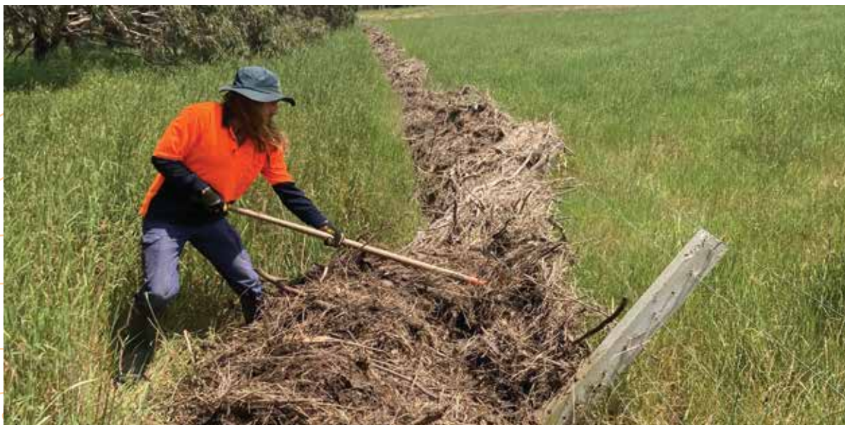
Below: The Glenelg Hopkins CMA works crew undertook significant flood recovery works with landholders after the 2022 floods. IMAGE: Glenelg Hopkins CMA.
