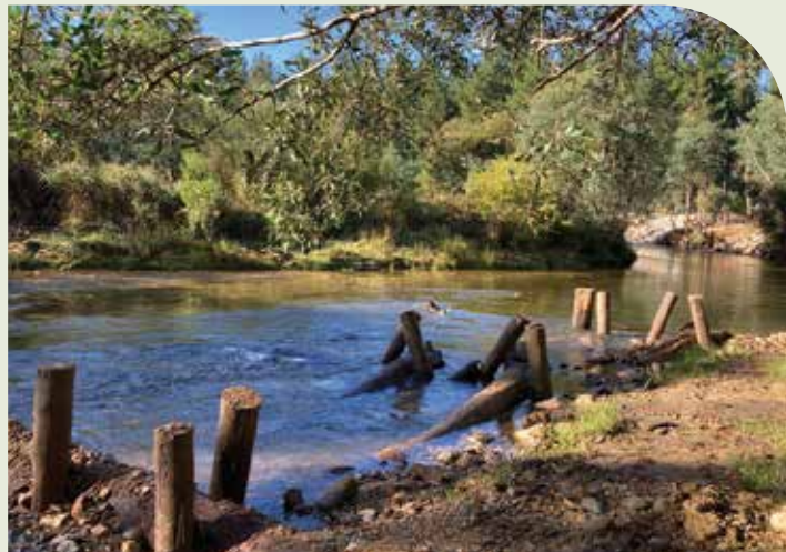
Installation of constructed log jams to create further habitat niches at Mayfly Rise. Image North East CMA.
