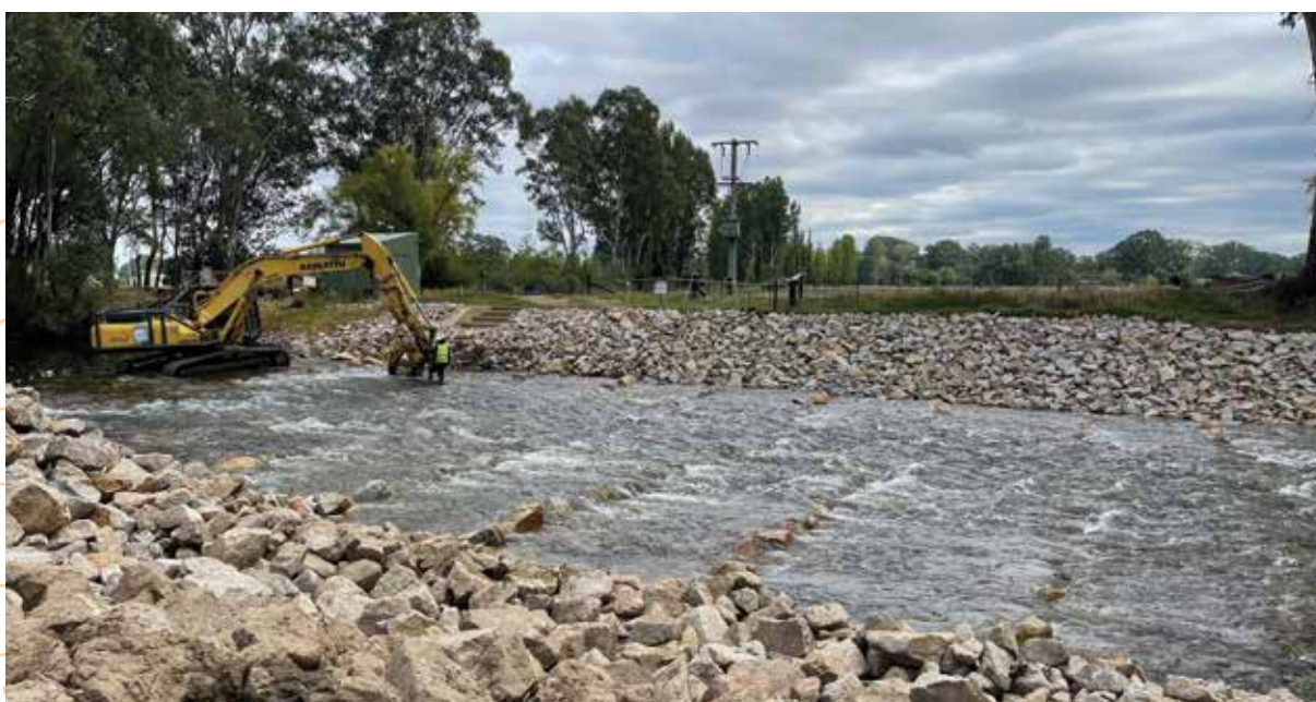
Below: A rock ramp fishway was constructed by North East CMA at the Tea Garden Weir on the Ovens River, near Everton, in partnership with Goulburn-Murray Water. Image Goulburn Murray Water.
