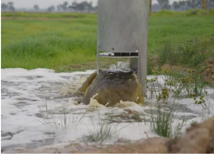
Figure 10, A pipe and riser outlet irrigating effluent water onto focus area 3, which had never had effluent applied to it.
