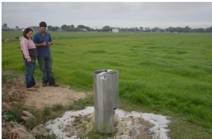
Steve and Jess on one of their trial paddocks with their new pipe and riser
