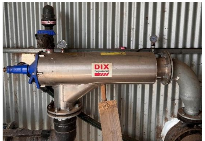
Figure 4, The secondary inline filter in situ in the pump shed.
