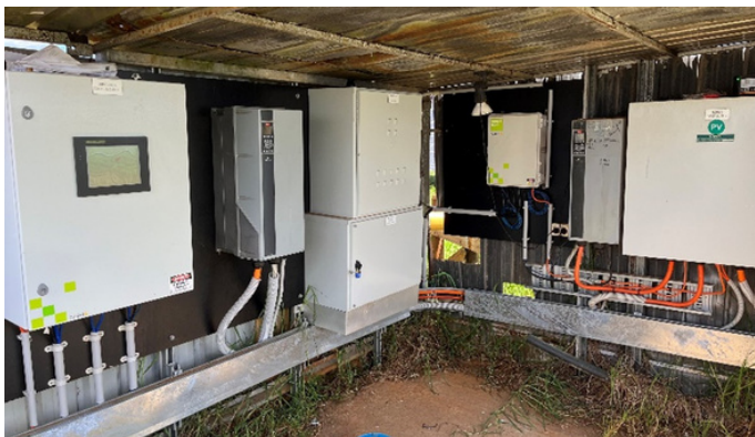
The AEI "SmartBox" and variable speed drives that run Wilandra Farm's fixed spray irrigation
